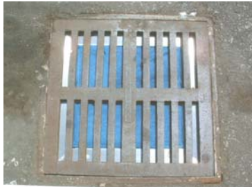
Storm Drain Basket Filter Installed
